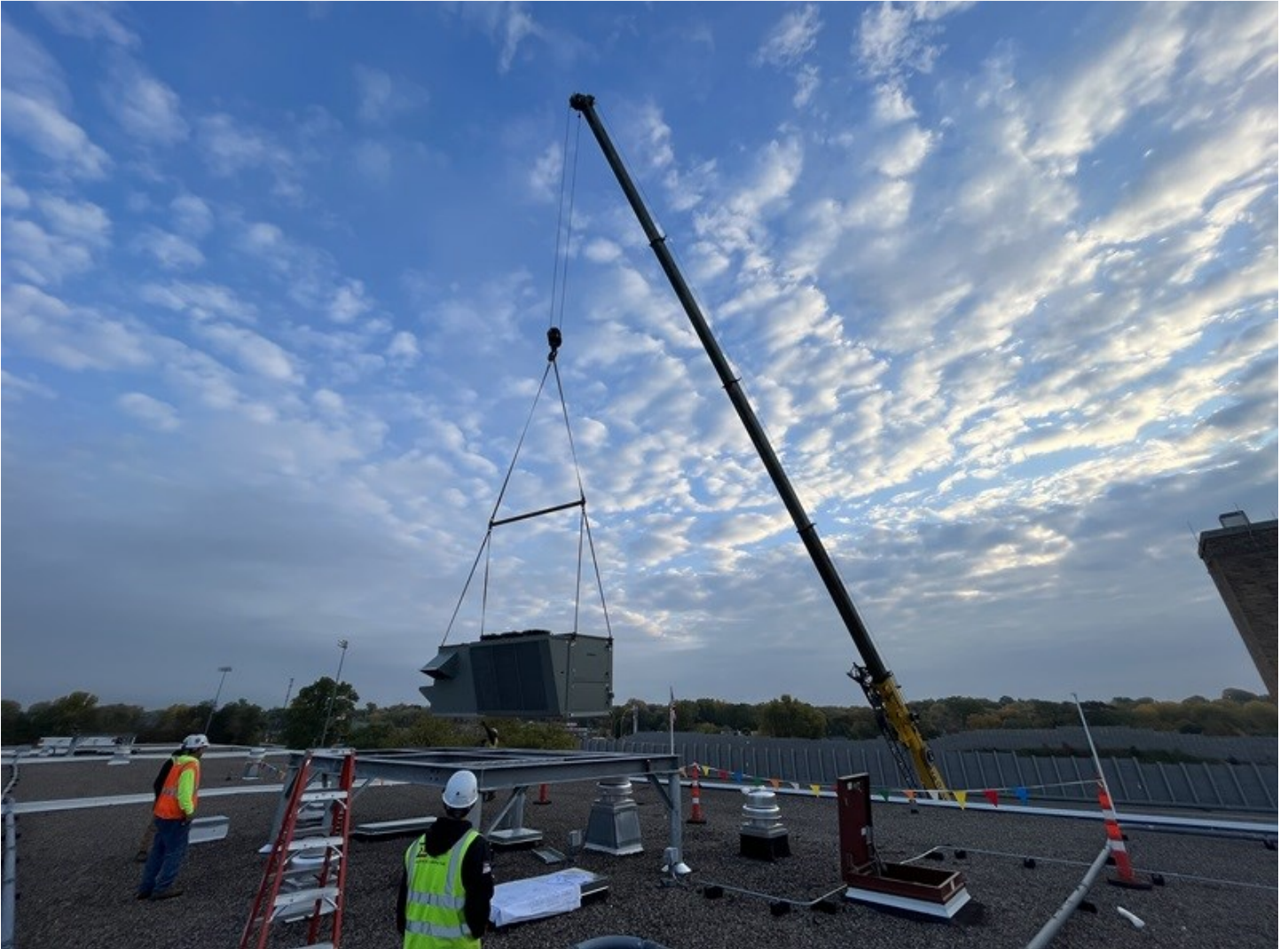
Rooftop air-handling units being lifted by a crane and set in place (October 2023)
